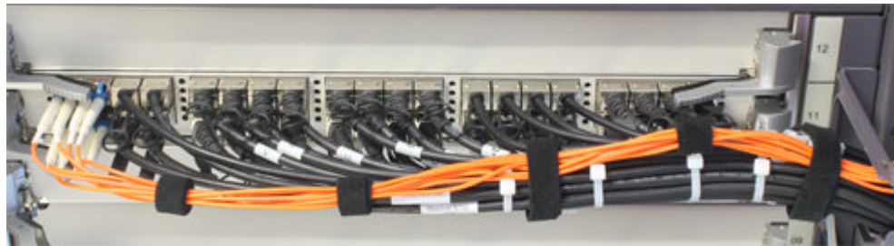
Figure 6-135 Optical fibers and SFP+ cables on the same card
