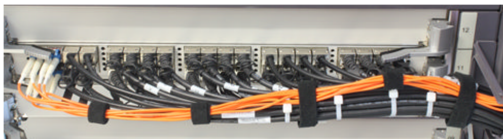
Figure 6-130 Arrangement of optical fibers and SFP+ cables
