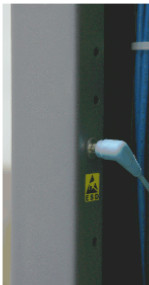
Figure 2-14 ESD jack in the middle of the N68E cabinet
