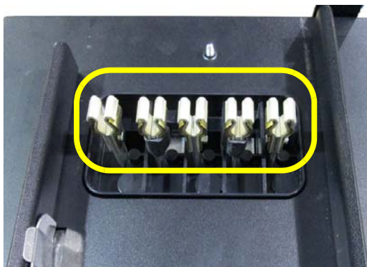
Figure 6: Inspect Plug-in Jaws
