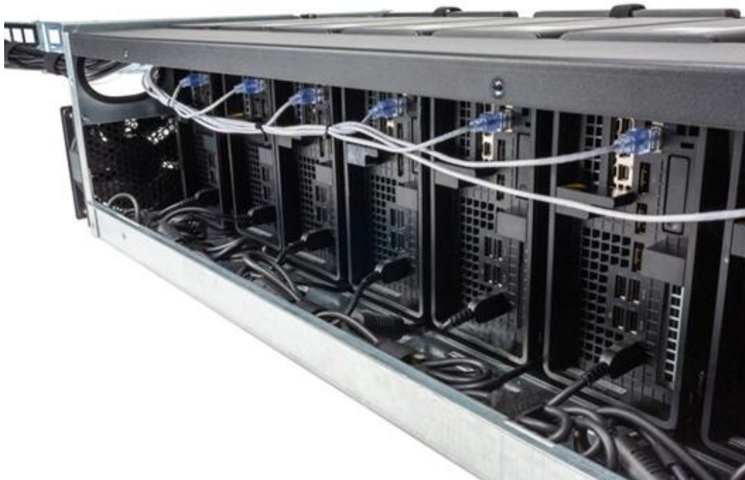
Figure 11 – HyperShelf Fully Populated with Ethernet and Power Cables Routed
